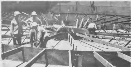
ROOF AND floor of a tank are built first; the floating roof is built inside and raised to the top when the tank is finished
